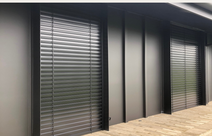
EV93D IN WINDOW SURROUND
